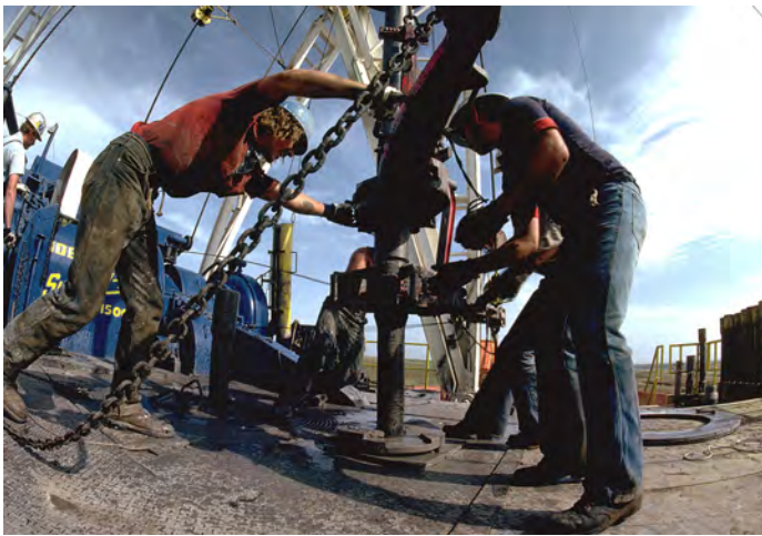
Developing domestic shale gas resources means additional jobs when wells are drilled, pipelines are constructed, and production facilities are built and operated.
