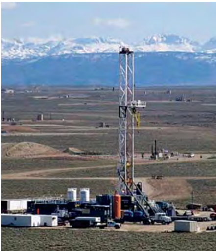
Shale drilling site in Wyoming. Photo: David Mott, U.S. Geological Survey Wyoming Water Science Center, http://pubs.usgs.gov/fs/2012/3049/FS12-3049_508.pdf
